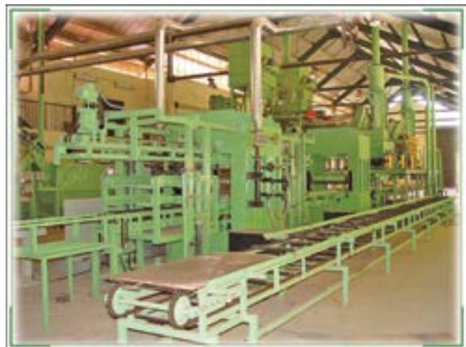
PARTICLE BOARD PLANT
