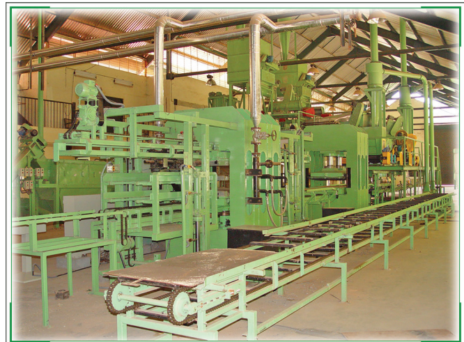
PARTICLE BOARD PLANT
